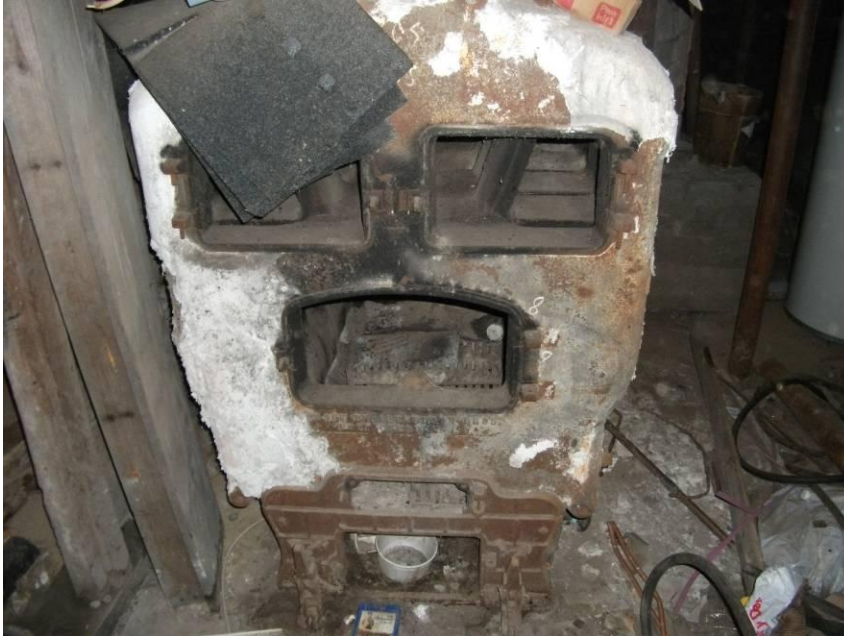
Picture 8 View of the out-of- service coal-fired furnace with potential asbestos containing insulation observed in the basement of the Inn.
