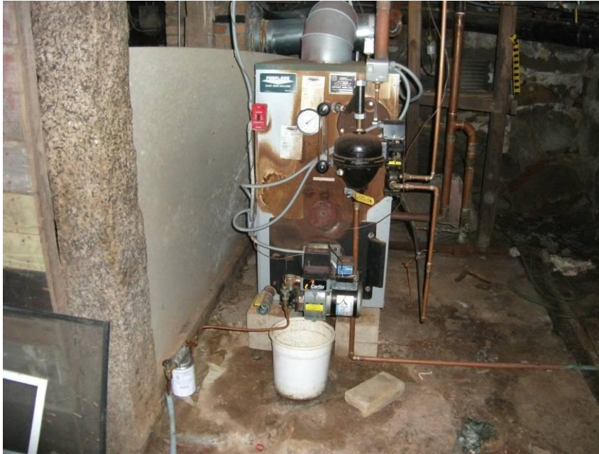
Picture 7 View of the No. 2 fuel oil-fire furnace observed in the basement of the Inn.
