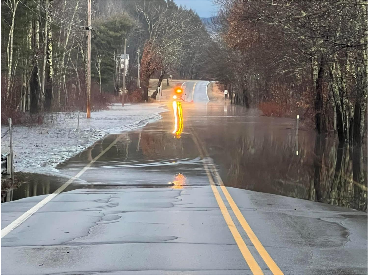
Flooding US Rte. 4 between Plains Road and Main St Dec. 2023
