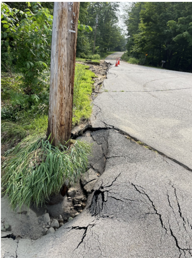
Water damage in Barnstead, NH 2023
