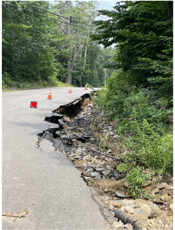
Water damage in Center Barnstead, NH 2023
