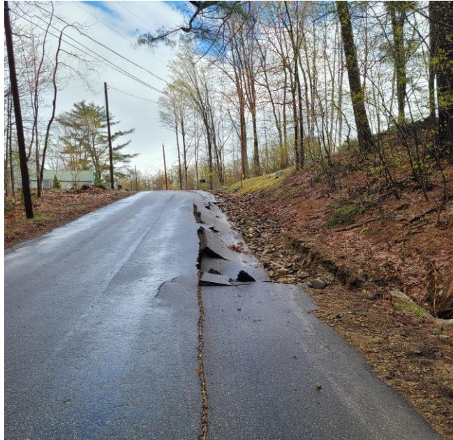
Shoulder washout due to flooding event on Lockes Hill Road in Gilford
