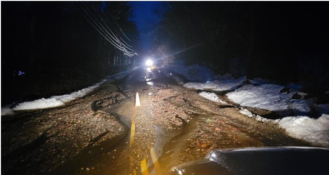
Flooding in Gilford due to December 2022 rainstorm
