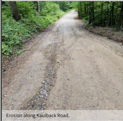
Erosion along Kaulback Road.
