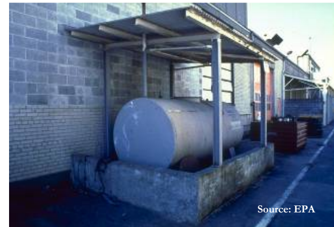
Aboveground storage tank for heating fuel
