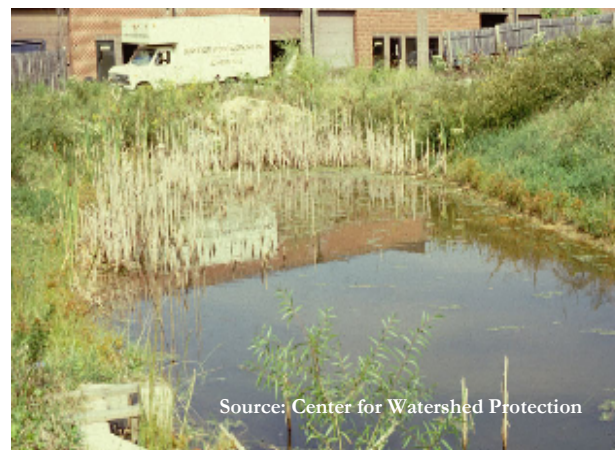
Infiltration basin clogged due to sediments
