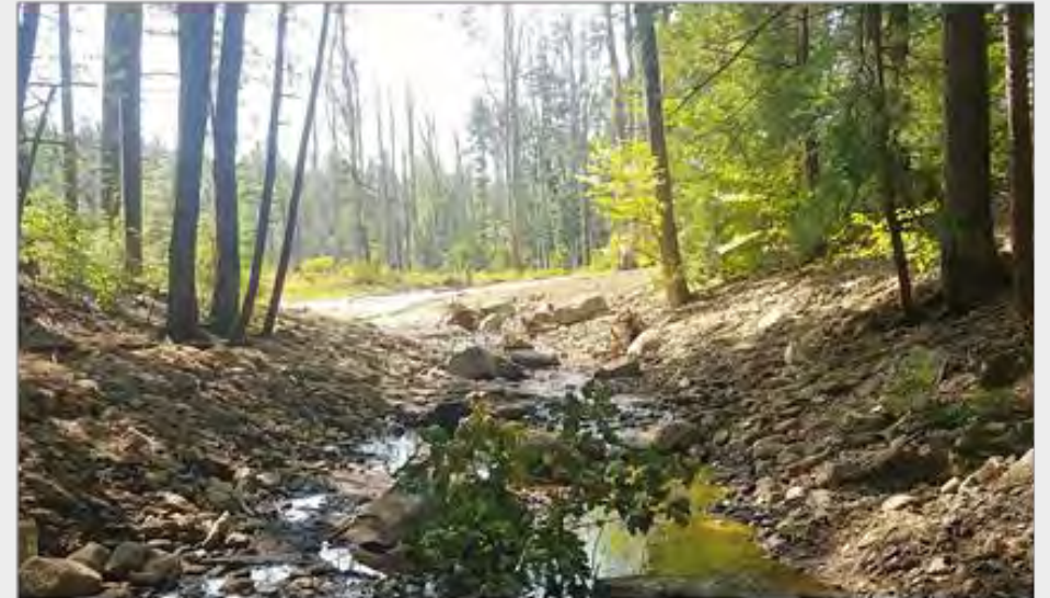
Photographs of Restoration of Brennan Brook in Frankestown through the removal of a dam (top). and restoration of aquatic and hydrologic connectivity completed in 2024 (bottom).
