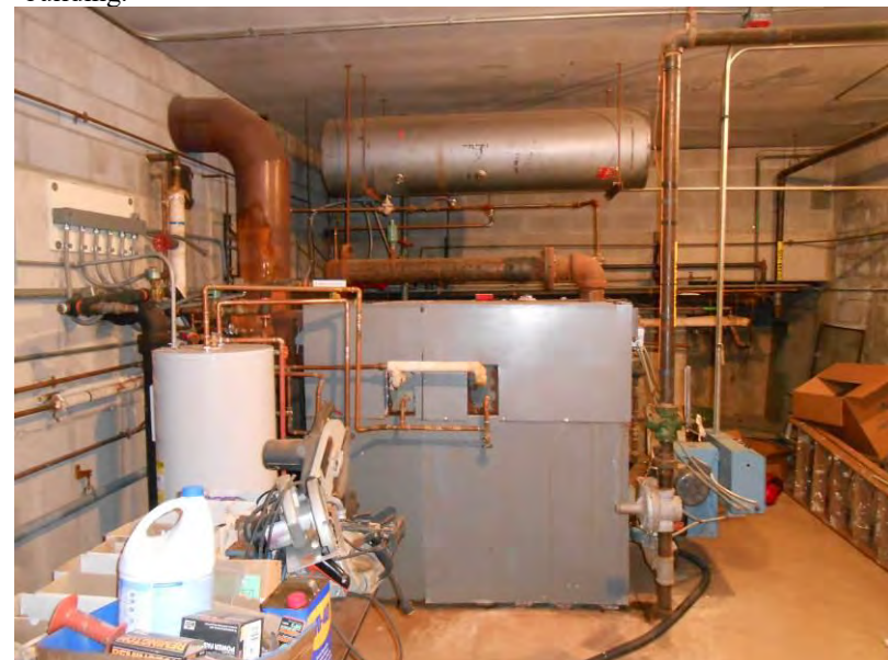
12. View of the boiler room in the Madeira office and warehouse building.
