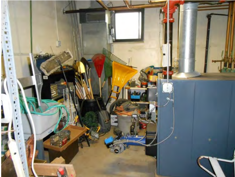
21. View of the current boiler room in the two-story building.
