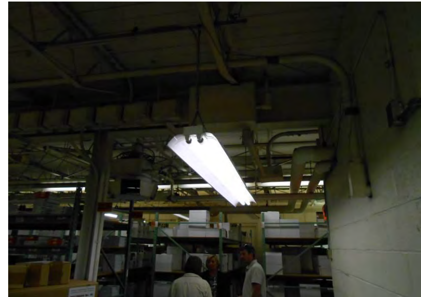
10. View of potential PCB-containing florescent light ballasts and suspect ACM pipe elbows in the warehouse of the Madeira office and warehouse building.
