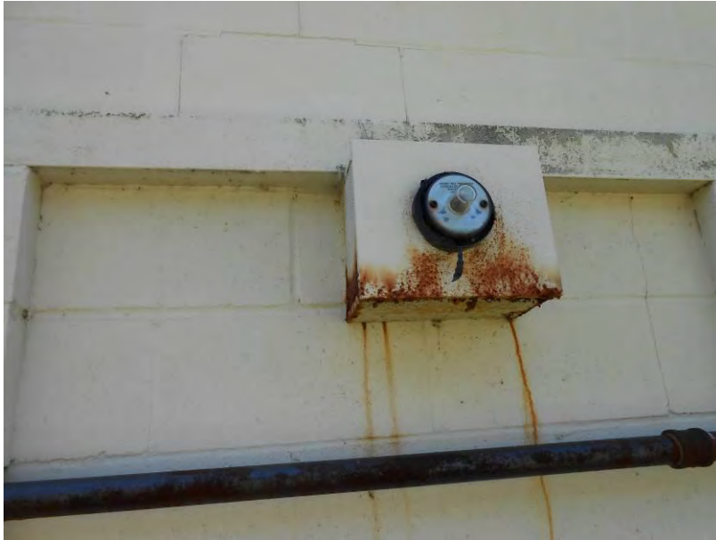
37. View of the potential overfill alarm of the suspected UST adjacent to the building.
