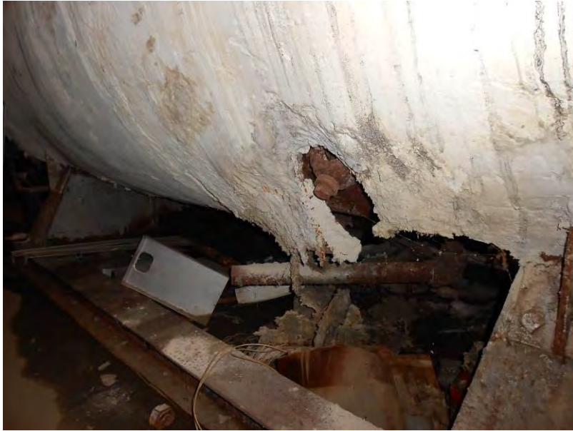
25. View of friable likely ACM in waste form.
