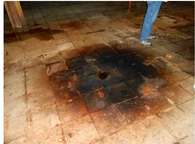
28. View of the water damage to the floor of the lower building.
