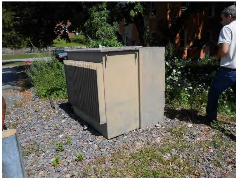
41. View of the electrical transformer for the Site.
