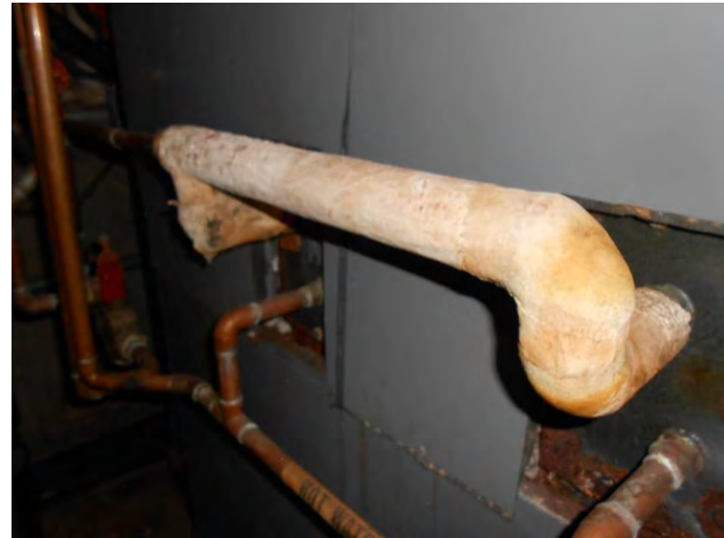
14. View of the suspect ACM in the boiler room of the Madeira office and warehouse building.
