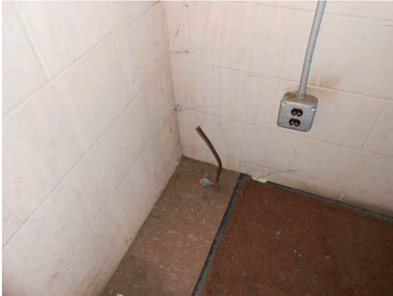
29. View of the copper pipe in the lower building.
