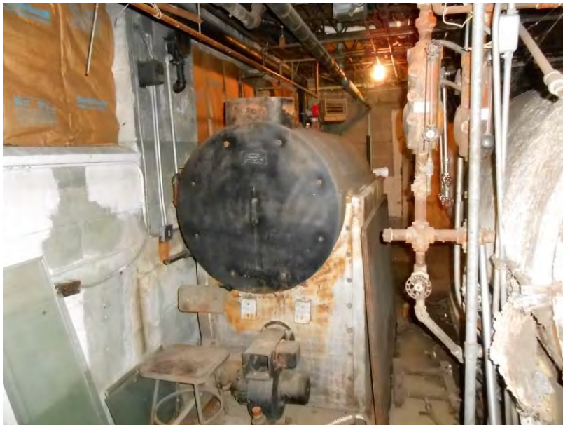
23. View of the second, smaller boiler in the former boiler room of the two-story building.
