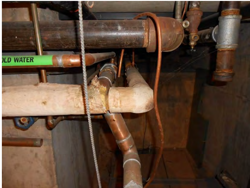
13. View of the suspect ACM in the boiler room of the Madeira office and warehouse building.
