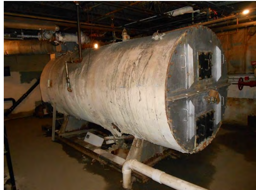
22. View of the large oil fired boiler in the former boiler room in the two-story building.
