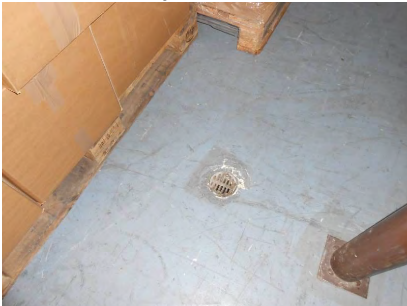
7. View of one of the two floor drains observed in the Madeira office and warehouse building.
