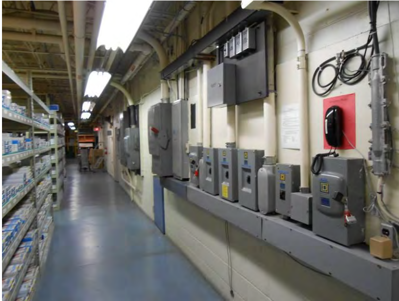
5. View of the first floor warehouse electrical equipment in the Madeira office and warehouse building.
