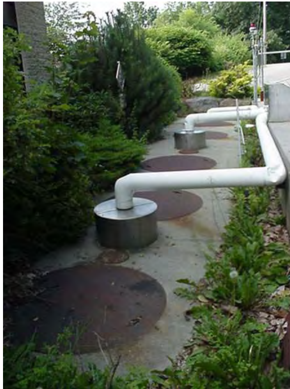
Photo 9 Underground Storage Tank (3 compartment)
