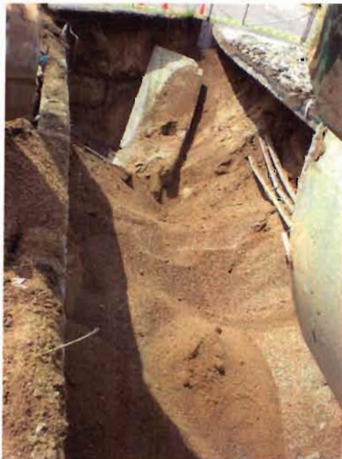
Photo 6 – View of 13,500-gallon UST basin.
