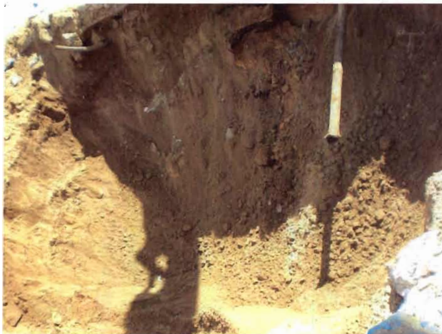
Photo 14 – View of 8,000-gallon UST basin.
