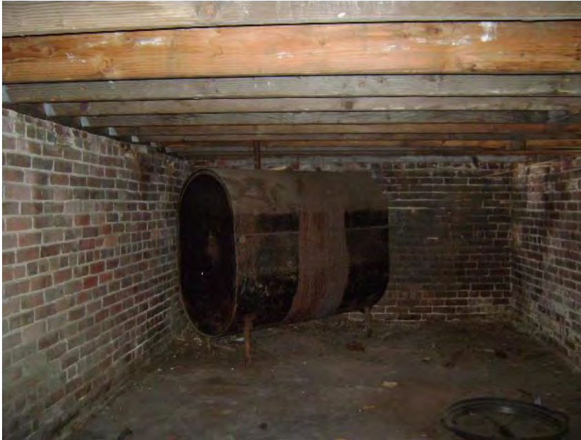
Picture 15 View of the 275- gallon AST observed in the southeast corner of the basement.
