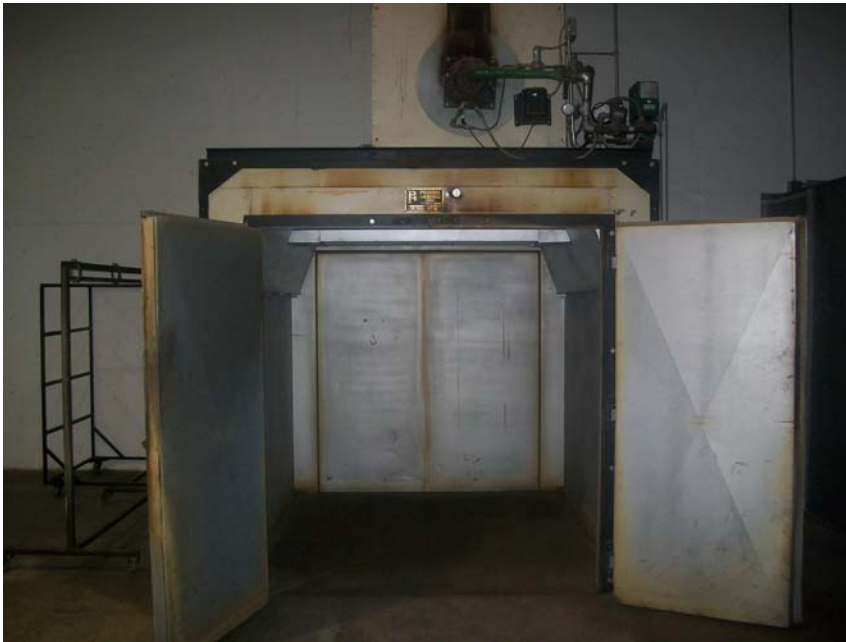
Picture 13 View of Central Powder Coating sandblasting booth.
