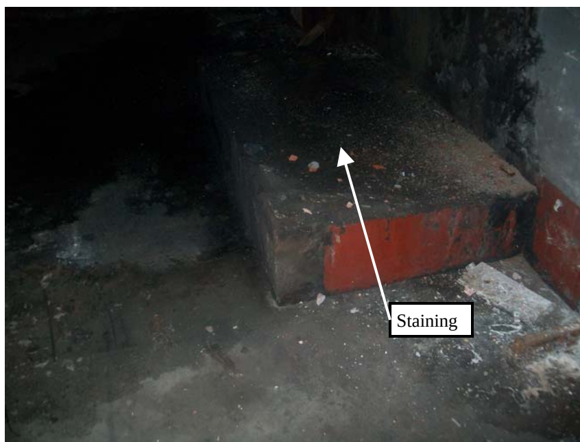
Picture 18 View of potential transformer pad in the bag room.
