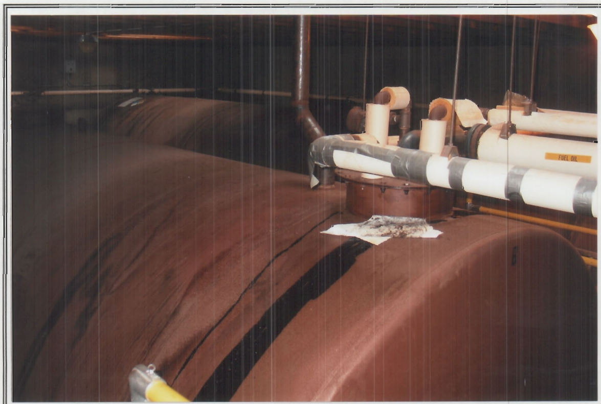
Photo 28. No. 6 fuel oil aboveground storage tanks in fuel oil storage building along Mechanic Street.
