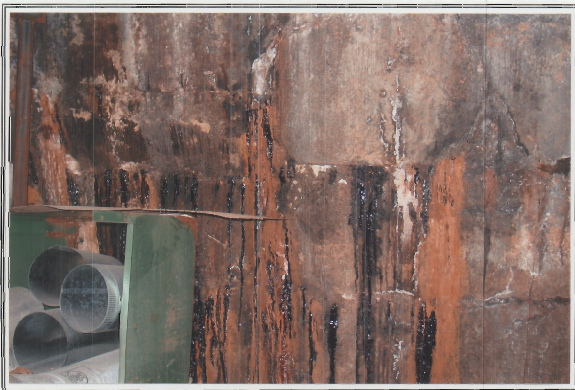
Photo 22. No. 6 fuel oil seeps along wall in storage room adjacent to boiler room.
