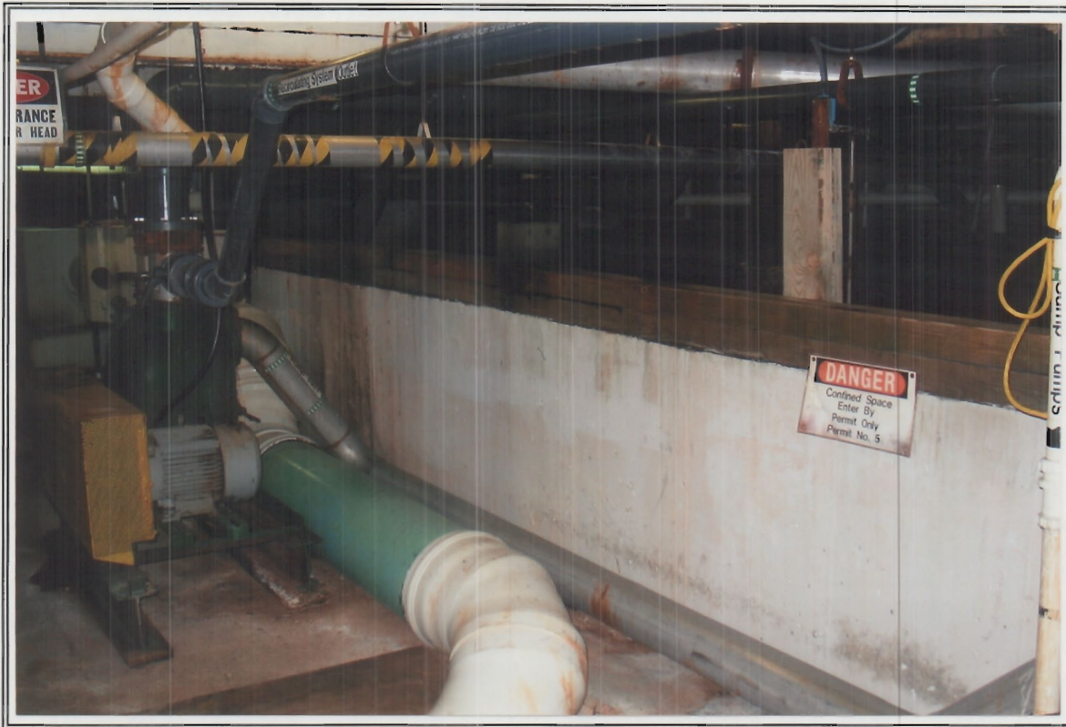
Photo 27. Wastewater pre-treatment plant. Blue and white piping is discharge to Ashland municipal sewer system.
