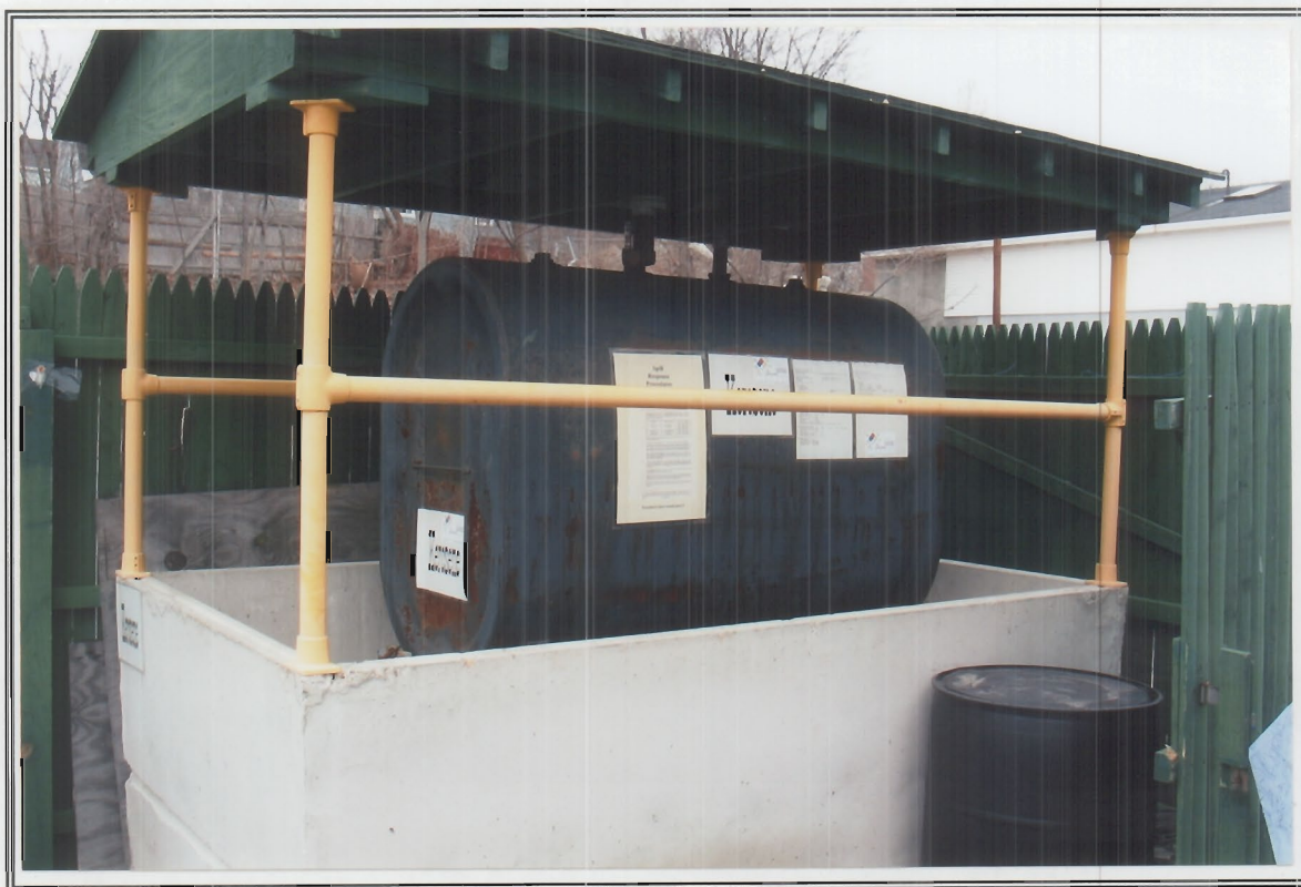
Photo 6. View of 275 gallon kerosene aboveground storage tank.
