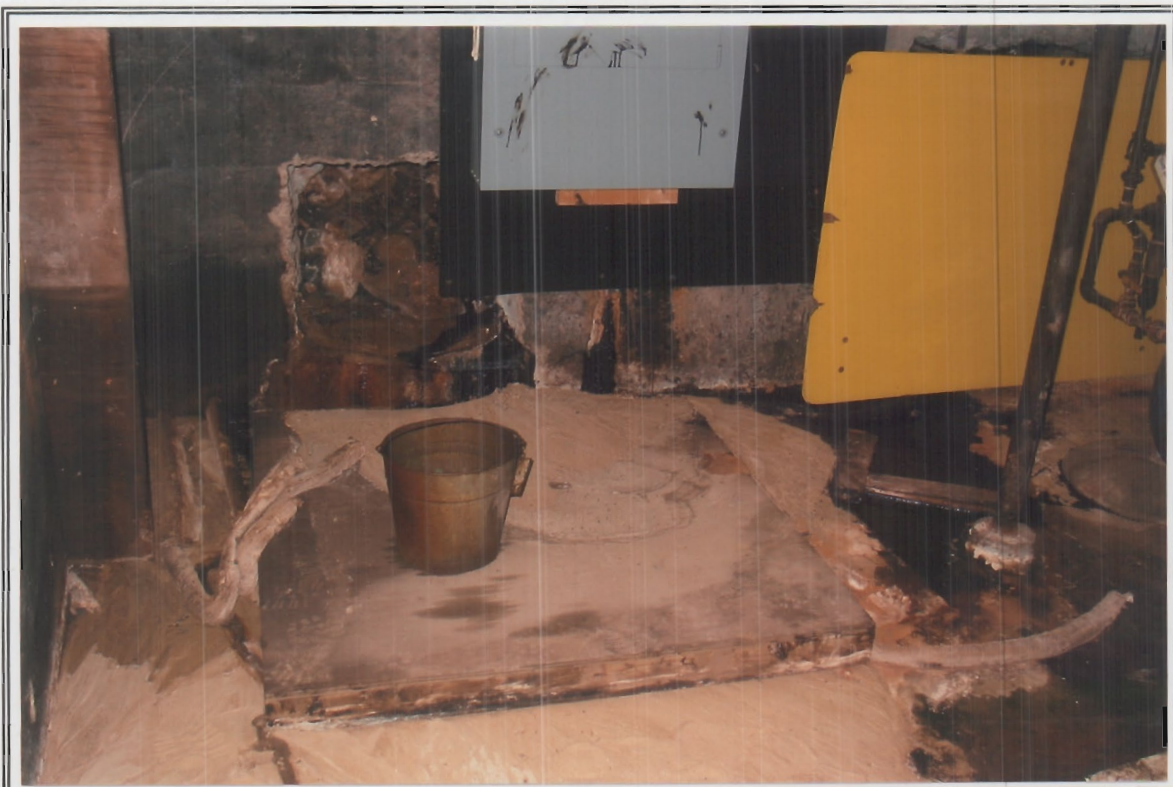
Photo 18. No. 6 fuel oil seep along back (northwest) wall of room below boiler room.
