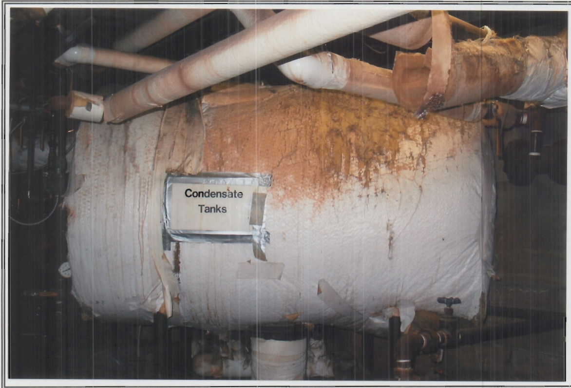
Photo 19. Condensate tank in room below boiler room.
