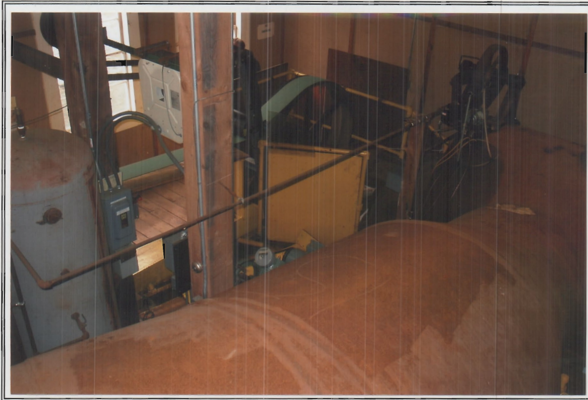
Photo 29. Penstock, water powered turbine and generator in Gate House building along Squam River, upstream of L. W. Packard building complex.
