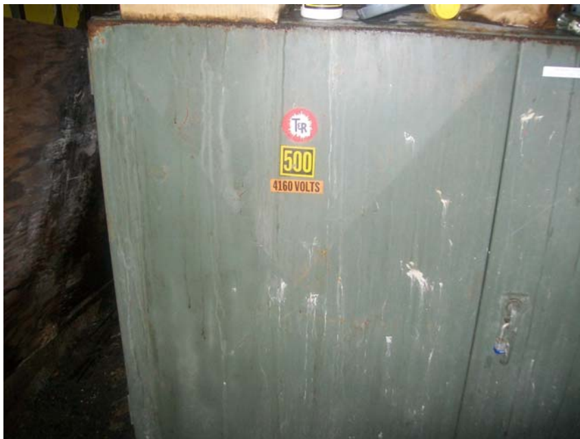
Picture 14 View of trans- former in Central Powder Coating area.
