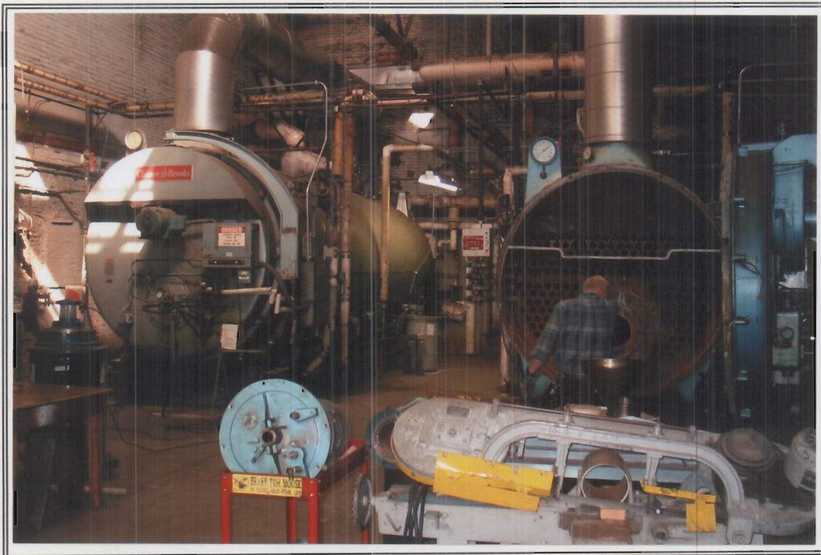
Photo 20. Steam boilers in boiler room fueled by no. 6 fuel oil.
