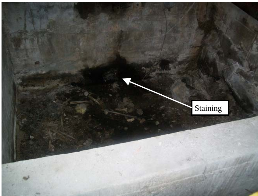
Picture 17 View of elevator shaft pit in southern basement with staining.
