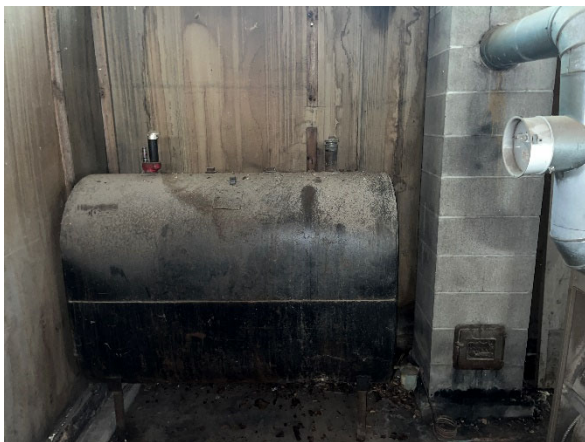
Photo 3: Half full heating oil tank in garage
