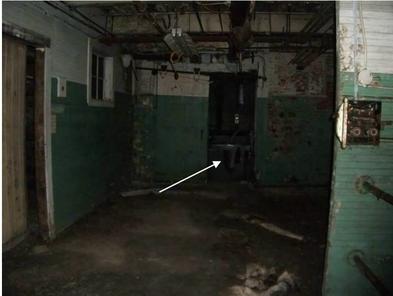
21. Location of boiler room at western end of the basement of Stanley Mill.
