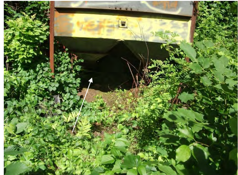
46. Possible metal dust beneath hopper on eastern side of Stanley Mill.
