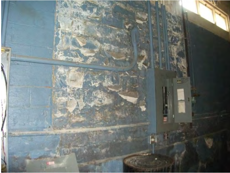
33. Peeling paint on wall of former Armory.
