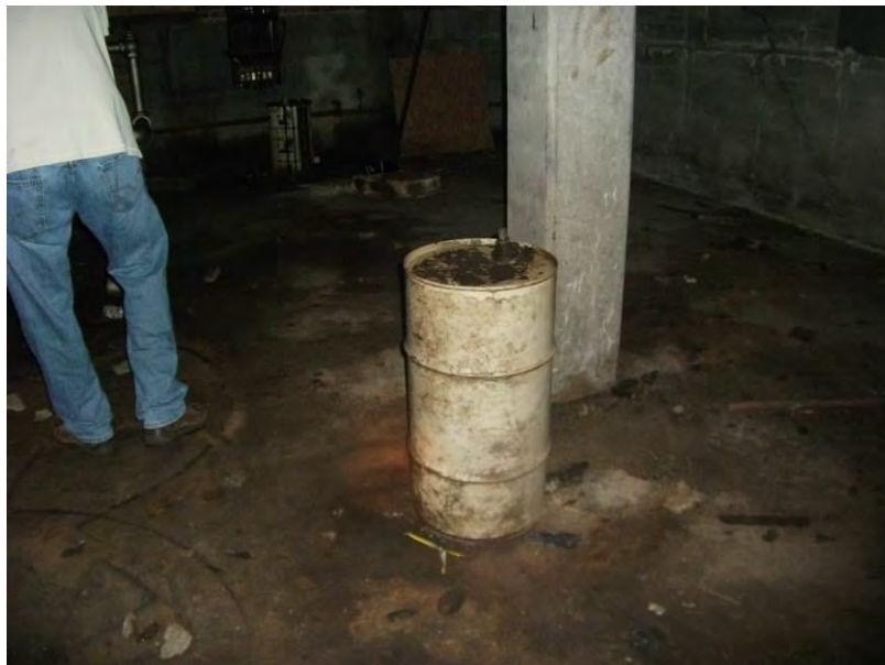
29. Drum of unknown material in northern basement portion of the Stanley Mill.
