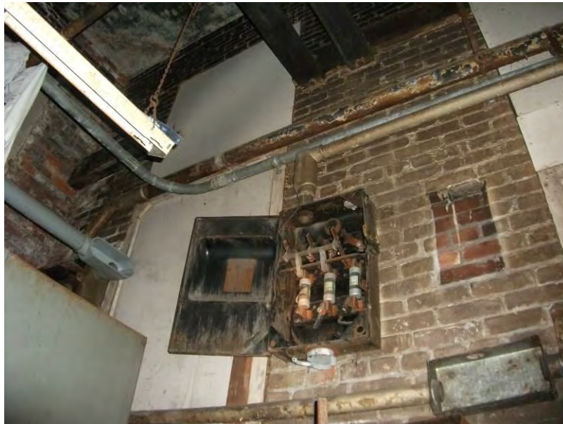
27. Electrical equipment in northeast corner of the Stanley Mill.
