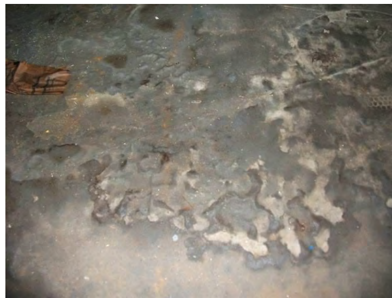
32. Peeling rubberized coating on floor of former Armory.
