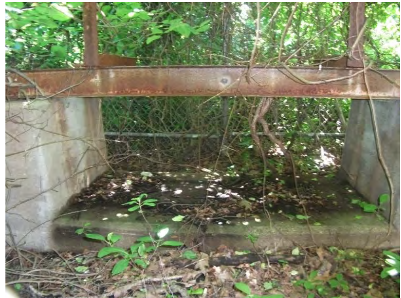
44. Former transformer area outside the northeast corner of the Stanley Mill. Note the staining on the concrete pad.
