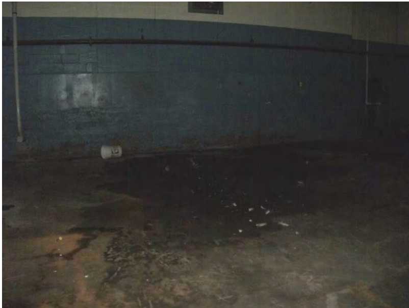
35. Staining near southern end the main room of the former Armory.
