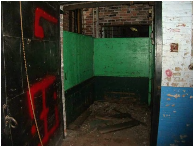
15. Elevator in southwest portion of the Stanley Mill.
