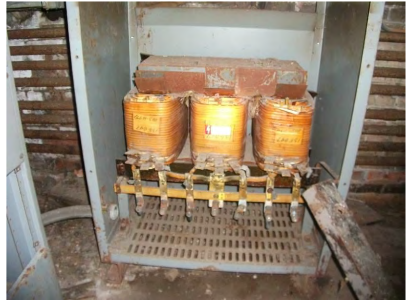
26. Electrical equipment in northeast corner of the Stanley Mill.
