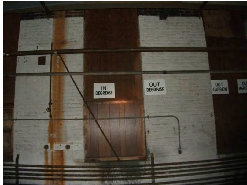
24. Image showing degreaser signs in northern portion of Stanley Mill.
