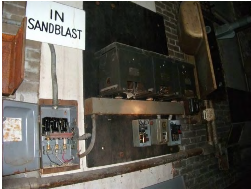
25. Electrical equipment in northeast corner of the Stanley Mill.
