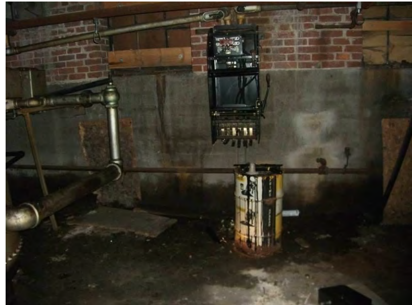
28. Electrical equipment in northeast corner of the Stanley Mill basement, also note drum of roofing tar.
