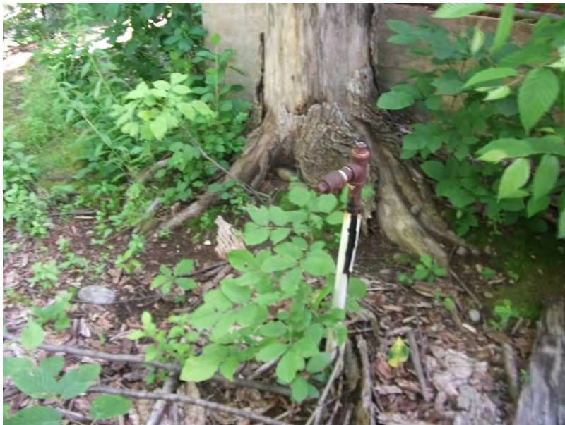
43. Disconnected piping coming from ground near northwest corner of Stanley Mill, 1 of 2 pipes.
