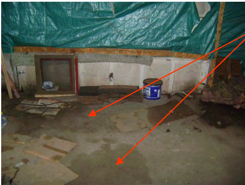
Picture 18 Representative view of staining observed in the garage bay.
