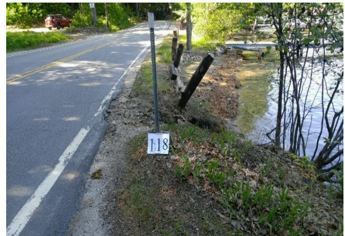
Rt. 113 along Cotton Cove suffers from complex runoff issues.
